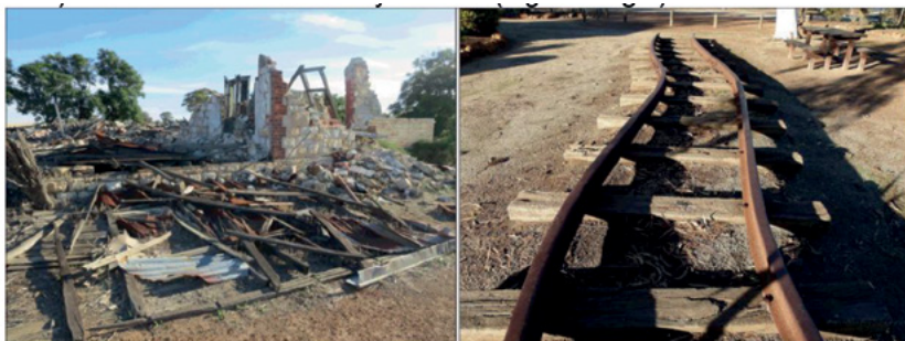
Fig. 4. Left: Building destroyed by the Meckering quake (Source http://www.ournauke-daustralia.com.au/tag/meckering/ ) Right: Buckled rails (Source: http://www.mingor.net/images-large/meckering-eq-buckled-rail-2011/ )
