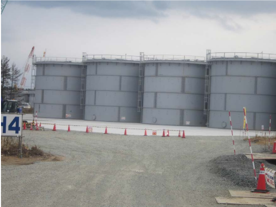
FIG. 25. Above ground tanks for storage of fresh water and concentrated salt water. Photograph courtesy of the Tokyo Electric Power Company (TEPCO) [41].
